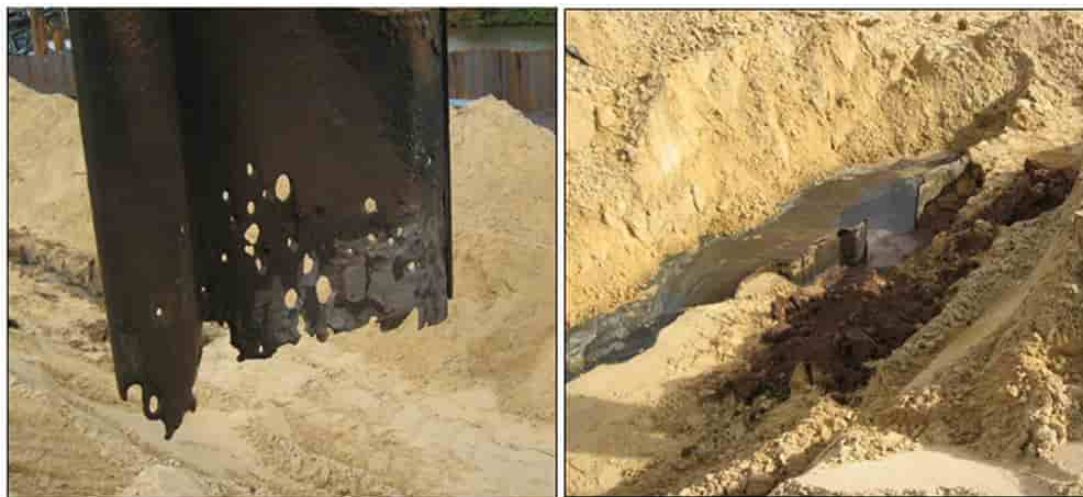
Severely corroded sheet pile
